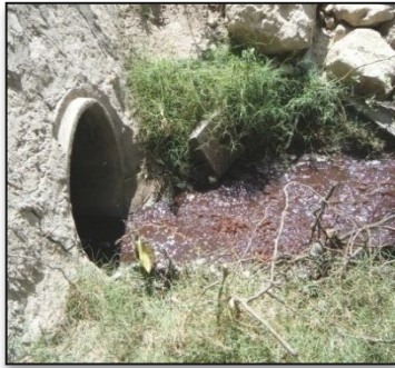
Photography 1. Direct discharge from FREASA to San Pedro river
